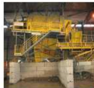
ashes/slag treatment plant in „Rinterzelt“
